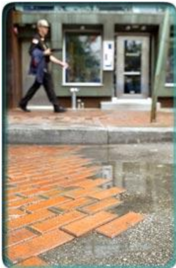
CASH IS CLAY: Bricks along the 200 block of Market Street lie in disrepair. Photo By: Mike Mergen
